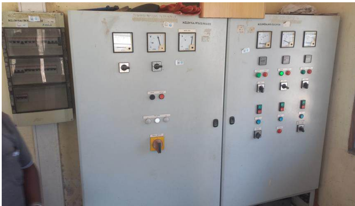
Mwanza South Pumping Station Motor Control Center (To be Replaced)
