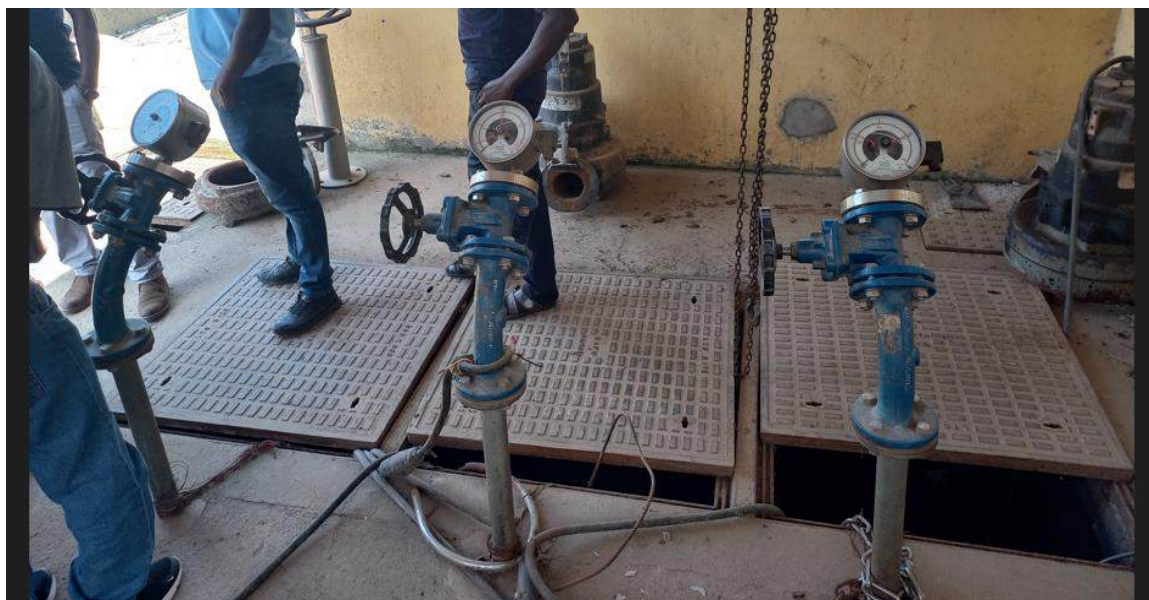
Kirumba Pumping Station Submersible Pumps (To be Replaced)
