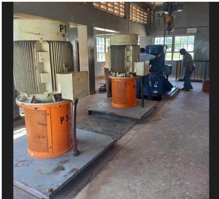
Central Pumping Station Pumps (To be Replaced)
