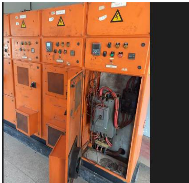
Central Pumping Station Motor Control Center (To be Retained)
